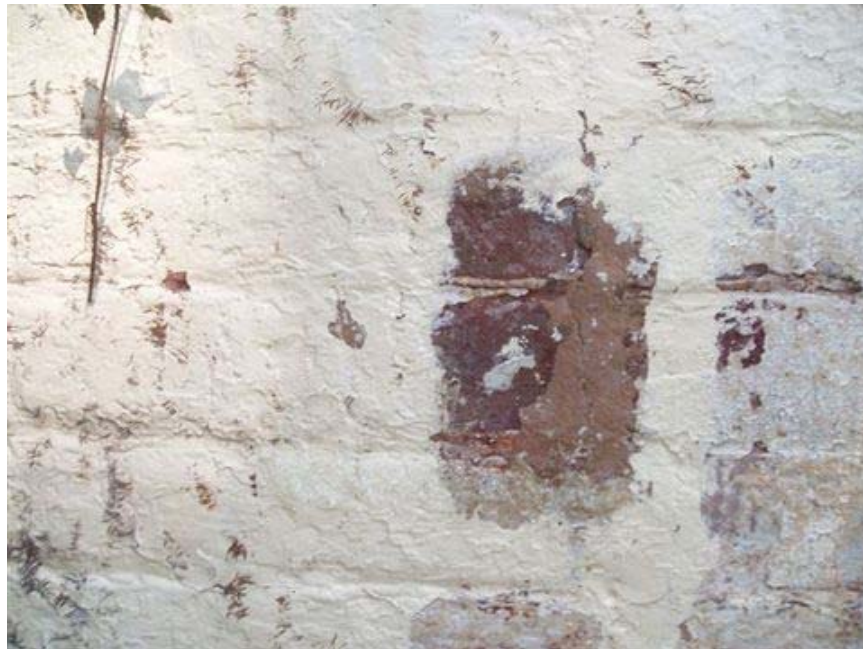
Figure 7: Area 3-S303, This product removed most paint layers after heavy wire brushing. It may be possible to use this product along with other mechanical removal means.
