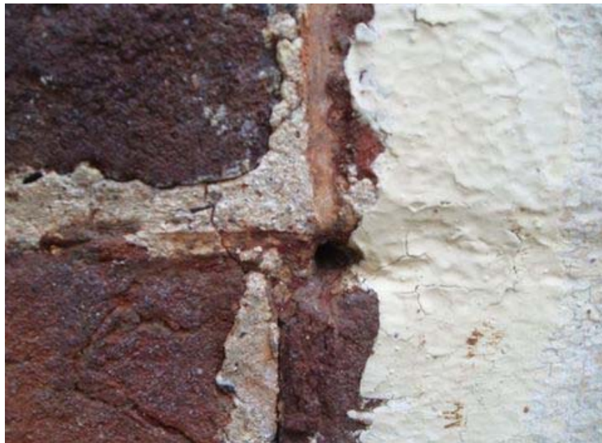
Figure 9: Detail of Area 5 showing poor mortar repairs that may be difficult to remove during restoration. Note feathering of mortar over brick faces.
