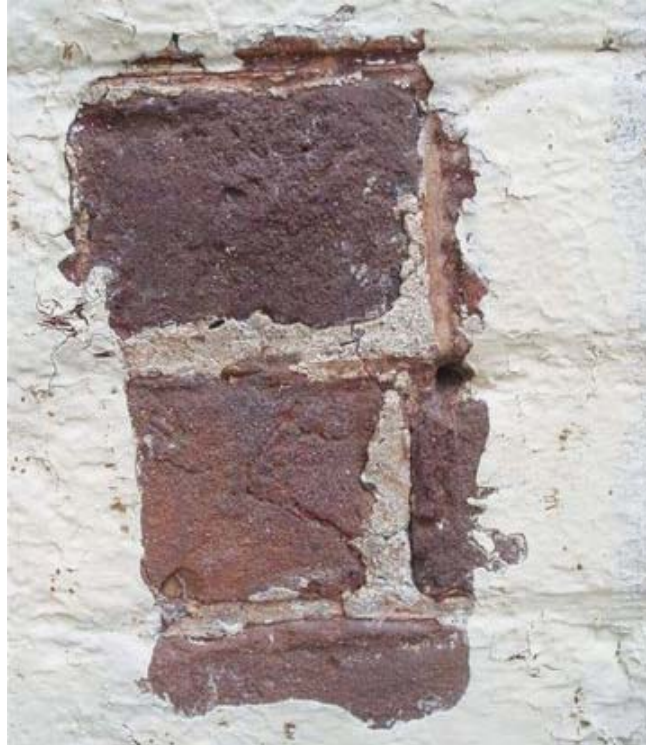
Figure 8: Area 5-Peel Away 1, this product worked best and removed all the paint layers. Some moderate wire brushing was necessary. Two applications of this product have been recommended to keep wire brushing to a minimum.
